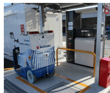
Hydrogen refueling system at Kosai Plant
