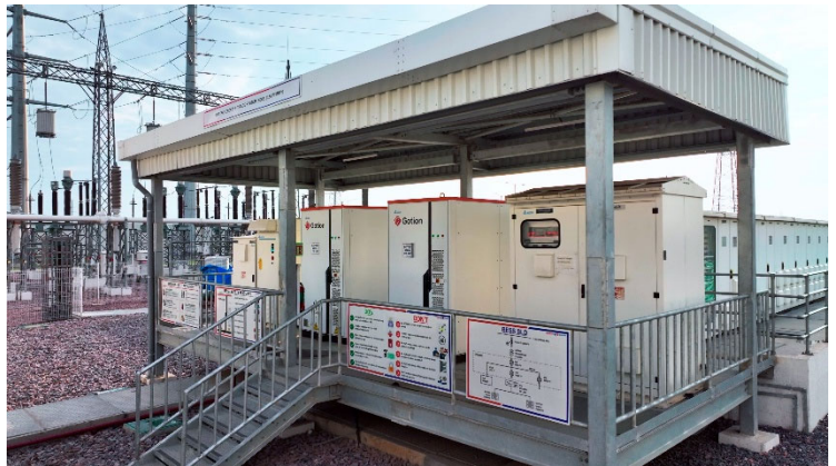
Battery energy storage system
