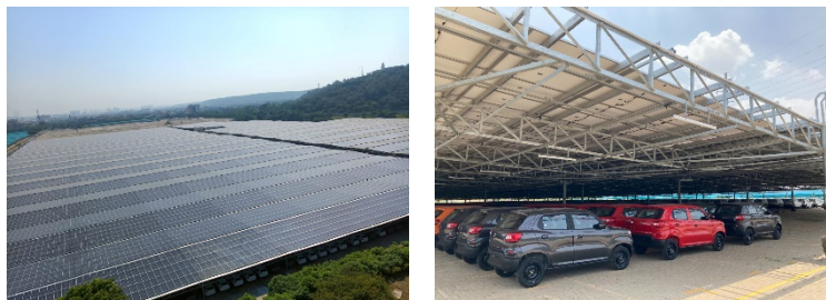
Solar panels established above the stock yard of Manesar Plant
