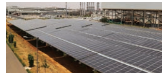
Solar Power Plant
