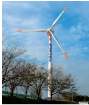
Wind power facility at Kosai Plant
